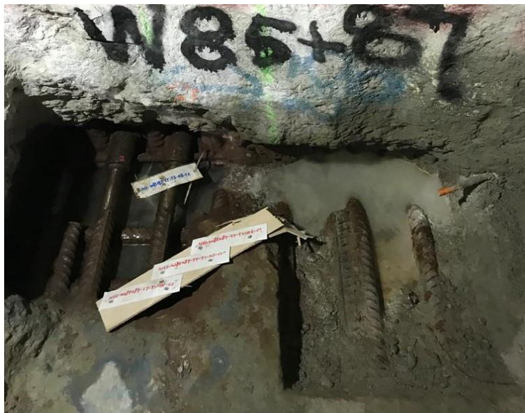
Figure 3-7 Water ponding at opening up location at NSL platform
