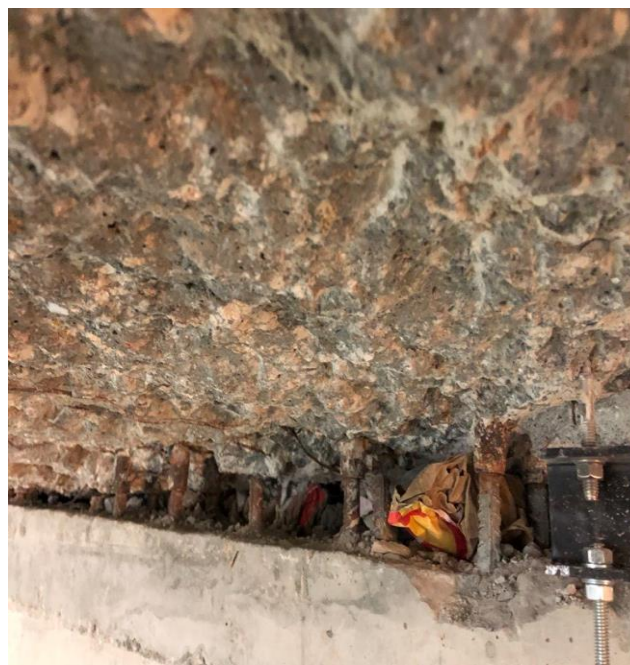
Figure 3-6 Gap between EWL slab and column
