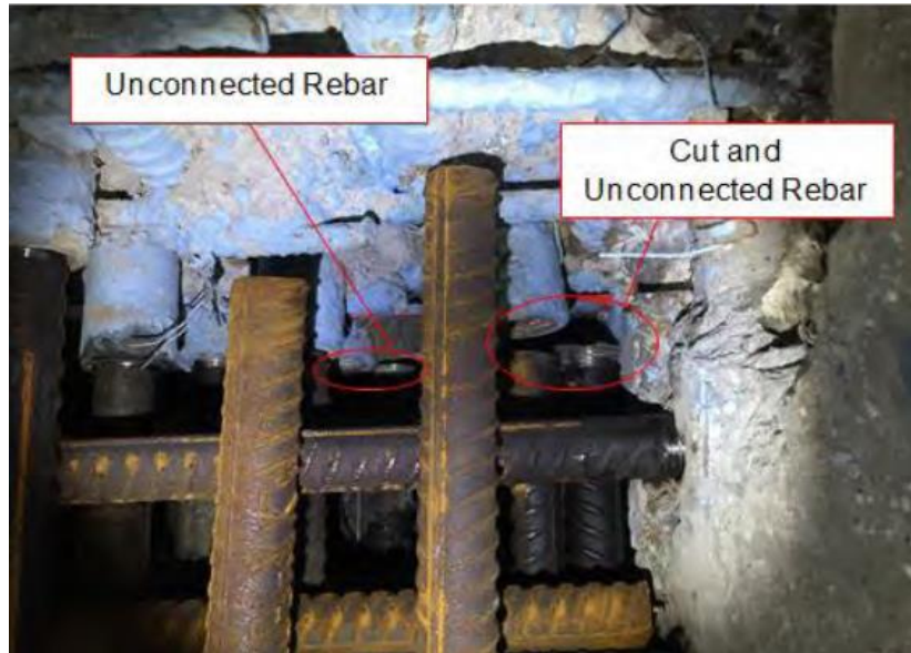
Figure 3-2 Site photograph at Panel EM100 in NCR 157 before rectification works
