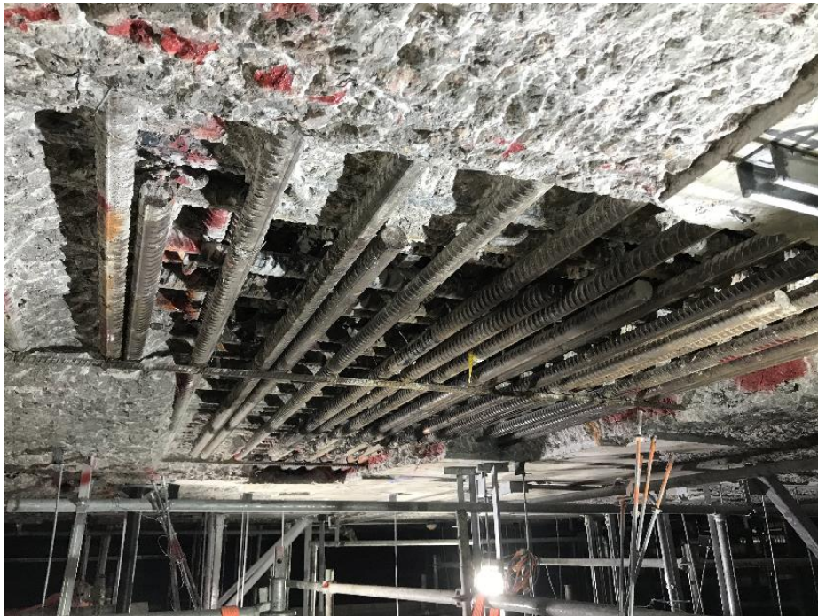
Figure 3-4 One of the deeper honeycombing areas after removal of honeycombed concrete at soffit of EWL slab
